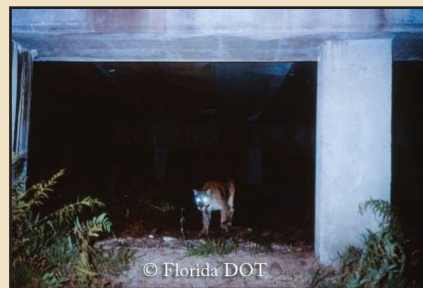
Culvert 50 meters from where F50 was struck by car. One of 3 within a half mile stretch of the site. No tall fencing present to funnel wildlife into safe passages.
