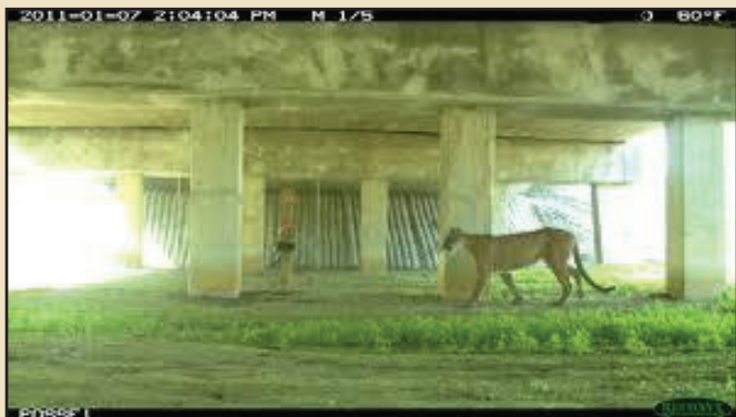
Bridge underpasses are preferred over pipe or box culverts (Beier 1995). In Beier's (1995) study, the majority of the transportation right-of-way crossings by dispersing juvenile mountain lions traveled under bridges.
